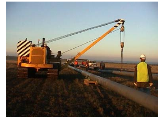
Above: Mitchell Oil & Gas Pty Ltd carried out the Pipeline Welding operations. The pipeline string was prefabricated and field joint coated behind the drill site in preparation for installation by the coedrill550 pipe pusher. Photo: E.Foley
