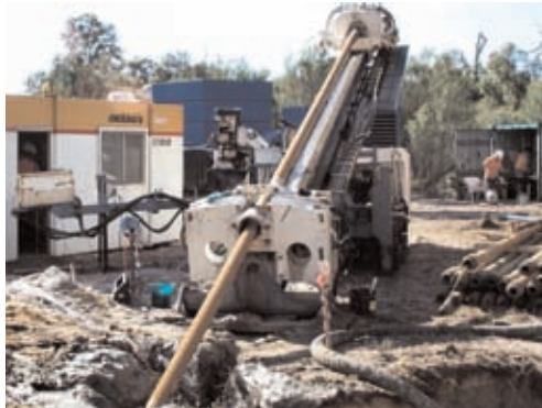
The 400 HDPE conduit will take raw waste water from the Australind-Eaton area to the new site at Kemerton, to undertake the river crossings.
